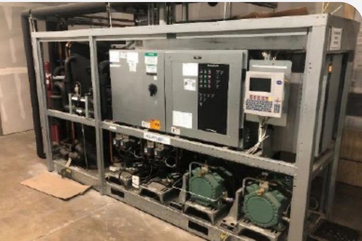
CO 2 (R-744) Refrigeration rack for the East Sacramento neighborhood Grocery Outlet store
