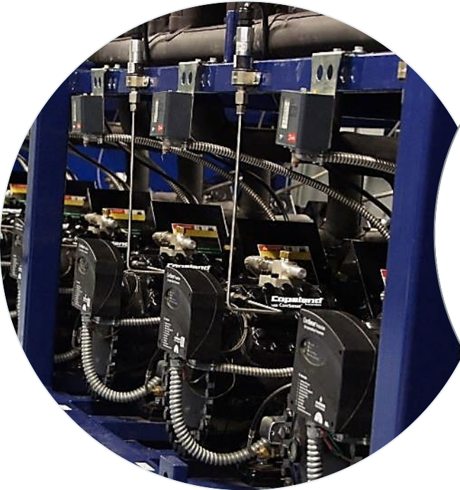
MT Compressor are rated for Minimum 1740 psig operating
