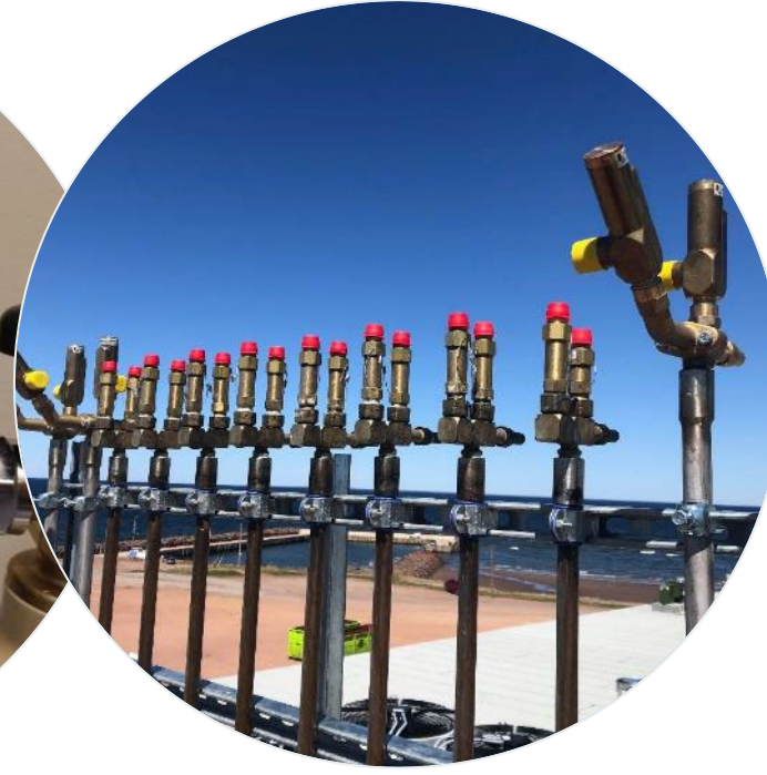
Verify if pressure-relief valves are installed in accordance with local building codes.
