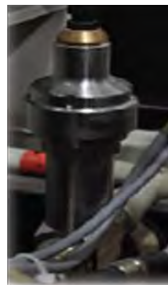
Flash gas by- pass valve
